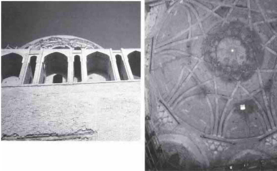
Fig. 16. Merv. Mausoleum of Sultan Sanjar, detail of the dome from outside (left) and inside (right). (Photo: Courtesy of I. Iskender-Mochiri.)
